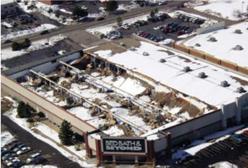
Figure 11. Collapsed roof of the large Bed, Bath, and Beyond store on south College Avenue in Ft. Collins, CO. The roof on this structure was replaced and the store re-opened several months later. Photo courtesy of Ron Phillips, City of Fort Collins.
